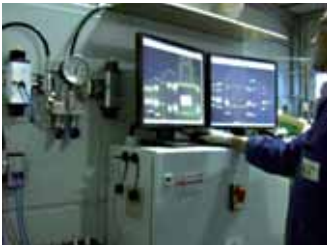
High pressure valves inspection-chamber
